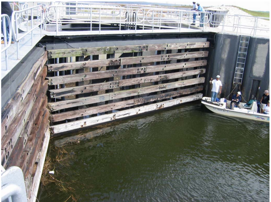
Picture 1: (Old) Bayou Bienvenue Sector Gate (New Orleans). 56 feet wide, 25 feet high. Picture by Tetra Tech.
